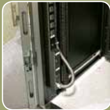
Power Distribution & Surge Protection
