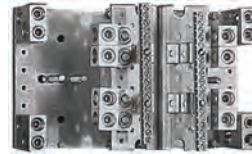
An Oversized Area is Provided for Neutral Connections with Ample Lugs for Ease of Installation
