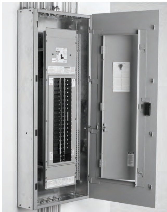
Trim Hanging on Surface Mounted Box
