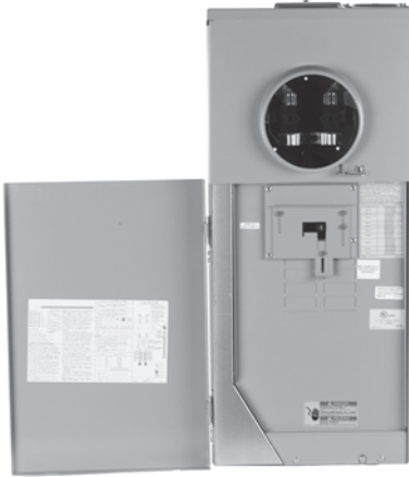
Meter Breaker with Interlock Cover
