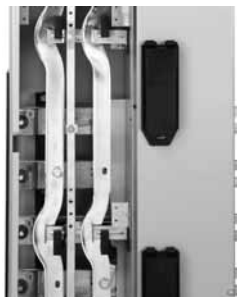
One-Piece Vertical Busbar
