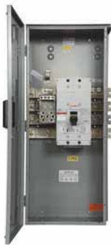
Main Circuit Breaker
