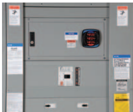
Custom Solar Switchboards
