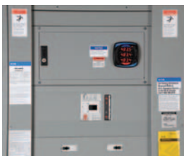
Custom Solar Switchboards
