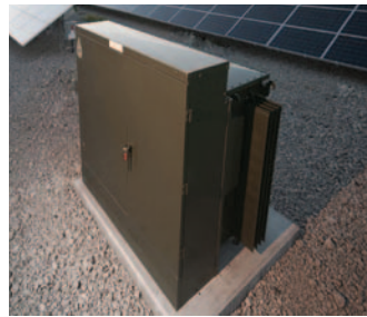
© 2010 Photo courtesy of Cooper Power Systems
