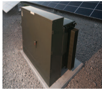
© 2010 Photo courtesy of Cooper Power Systems
