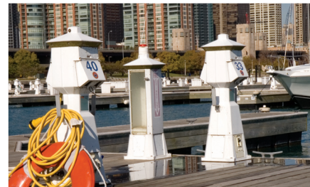
marine shore-power and dock lighting
