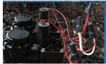
irrigation and sprinkler systems
