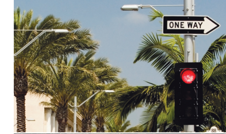
traffic signal controls
