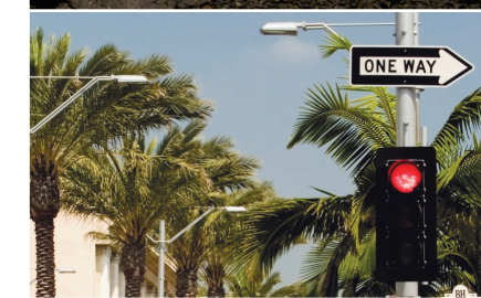
traffic signal controls
