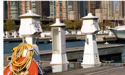
marine shore-power and dock lighting
