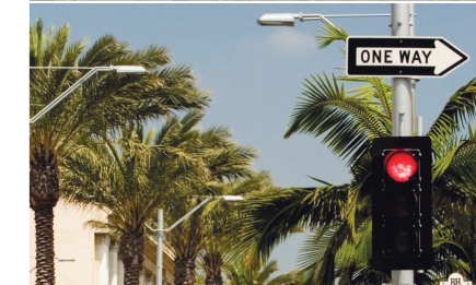
traffic signal controls
