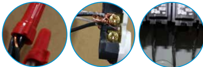
Improper solid wire connection.
