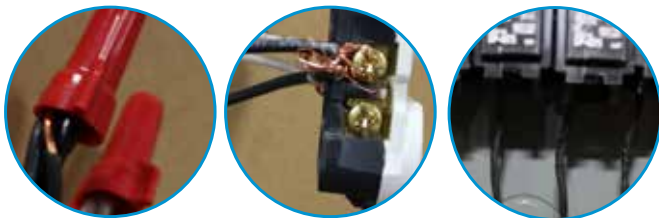
Improper solid wire connection.
